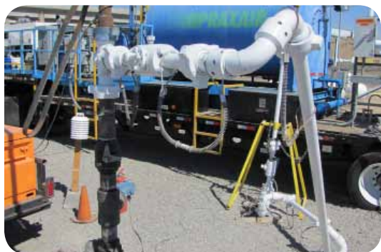
Pipeline infrastructure for injecting CO 2
